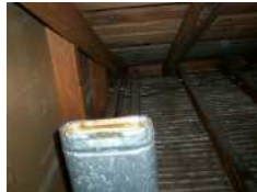
Heating vent terminating in the attic
