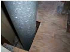
Insufficient clearance between hot vent and combustibles
